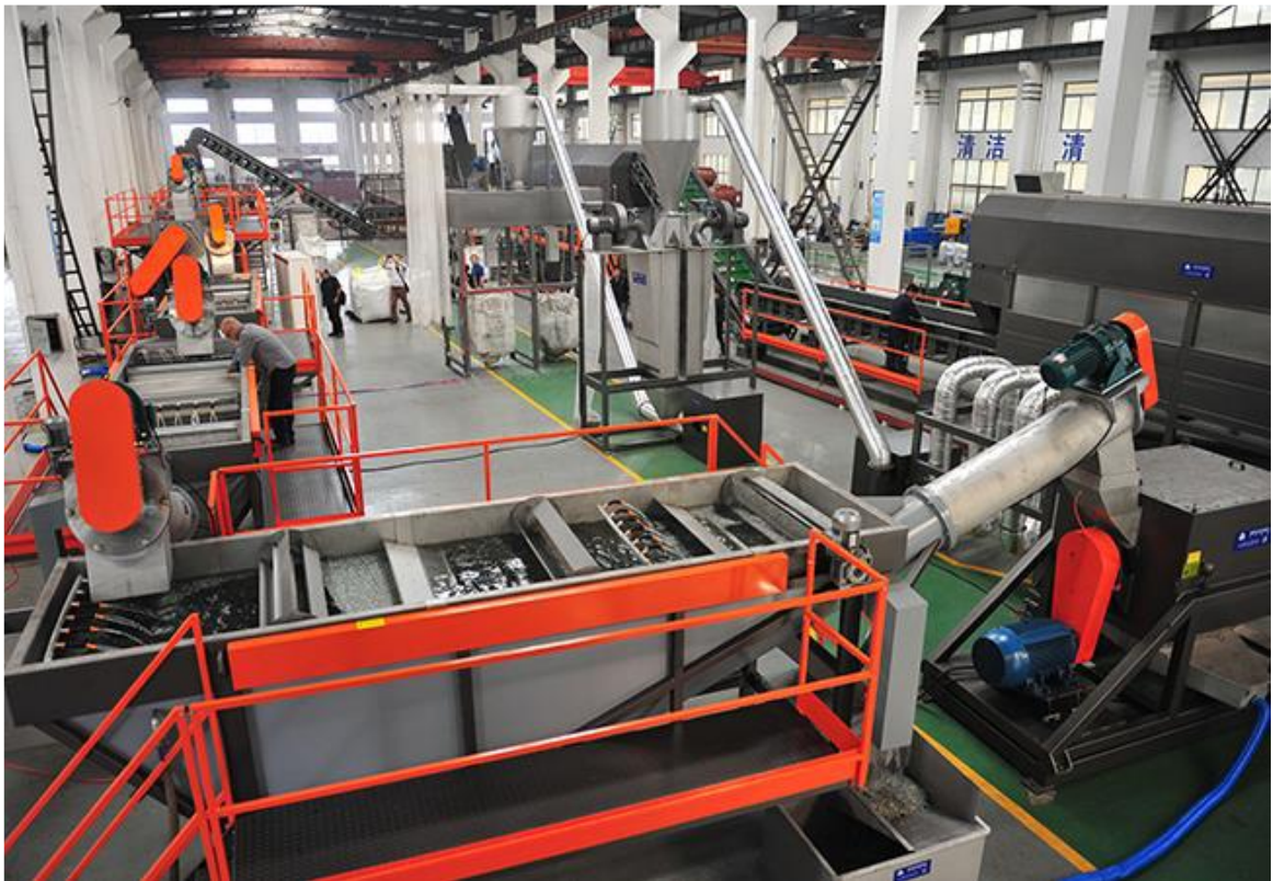
Figure 5 - Example of PET bottle washing and waste lines (Beier Machinery) Figure A.9 provided in the EIS by GHD (2022).
