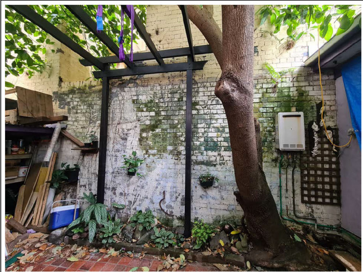
Figure 21: Photograph of the existing southern wall along the boundary between No. 6-8 Woodburn Street and No. 9 Woodburn Street. I request that this wall be retained to the boundary in this location and incorporated into the new construction of the proposed ground floor commercial space. If it is not possible to retain this wall, I request that the new wall be the same quality face brick as used elsewhere in the development.
