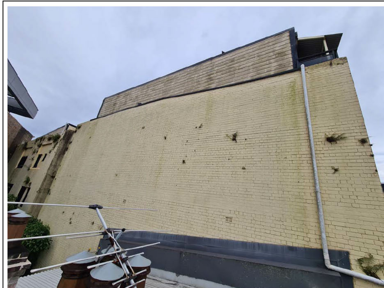
Figure 34: Photo showing the extent of the already imposing brick wall to the southern boundary of No. 6-8 Woodburn Street. I object to the proposed paint finish and colour to this wall due to concerns about quality of the building materials and the likely hood that finishes to this façade will not receive maintenance over time (as is evidenced in the existing situation where maintenance to this façade is not carried out because of difficulties with access). I request that the material used for the walls of the façade match the rest of the development, being a high-quality face brick.
