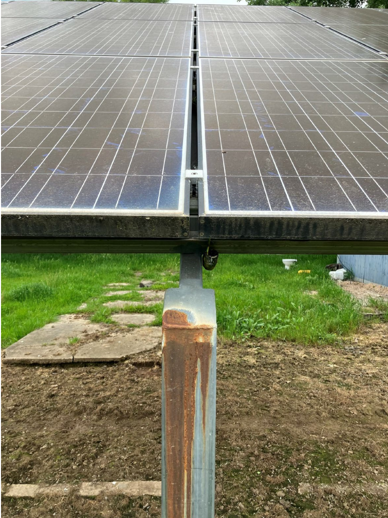
Run off corroding galvanised post
