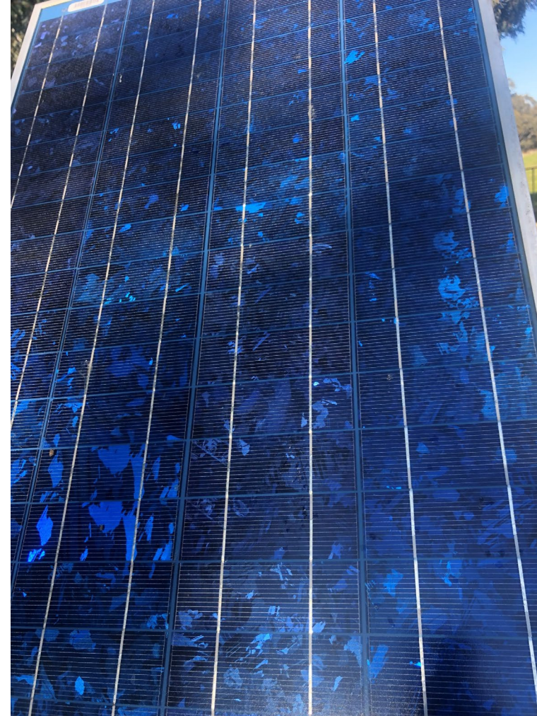
Solar panel breaking down after 10 years
