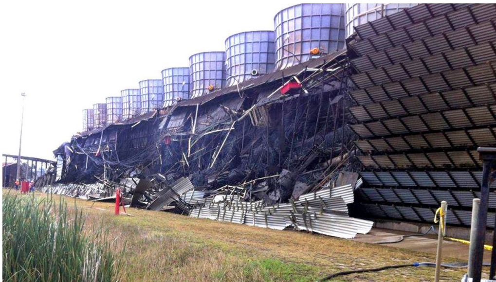
Wallerawang cooling tower collapse shown below. Water salinity may have been factor. [The cooling towers for Mt Piper Power Station are understood to be made of more durable materials.]
