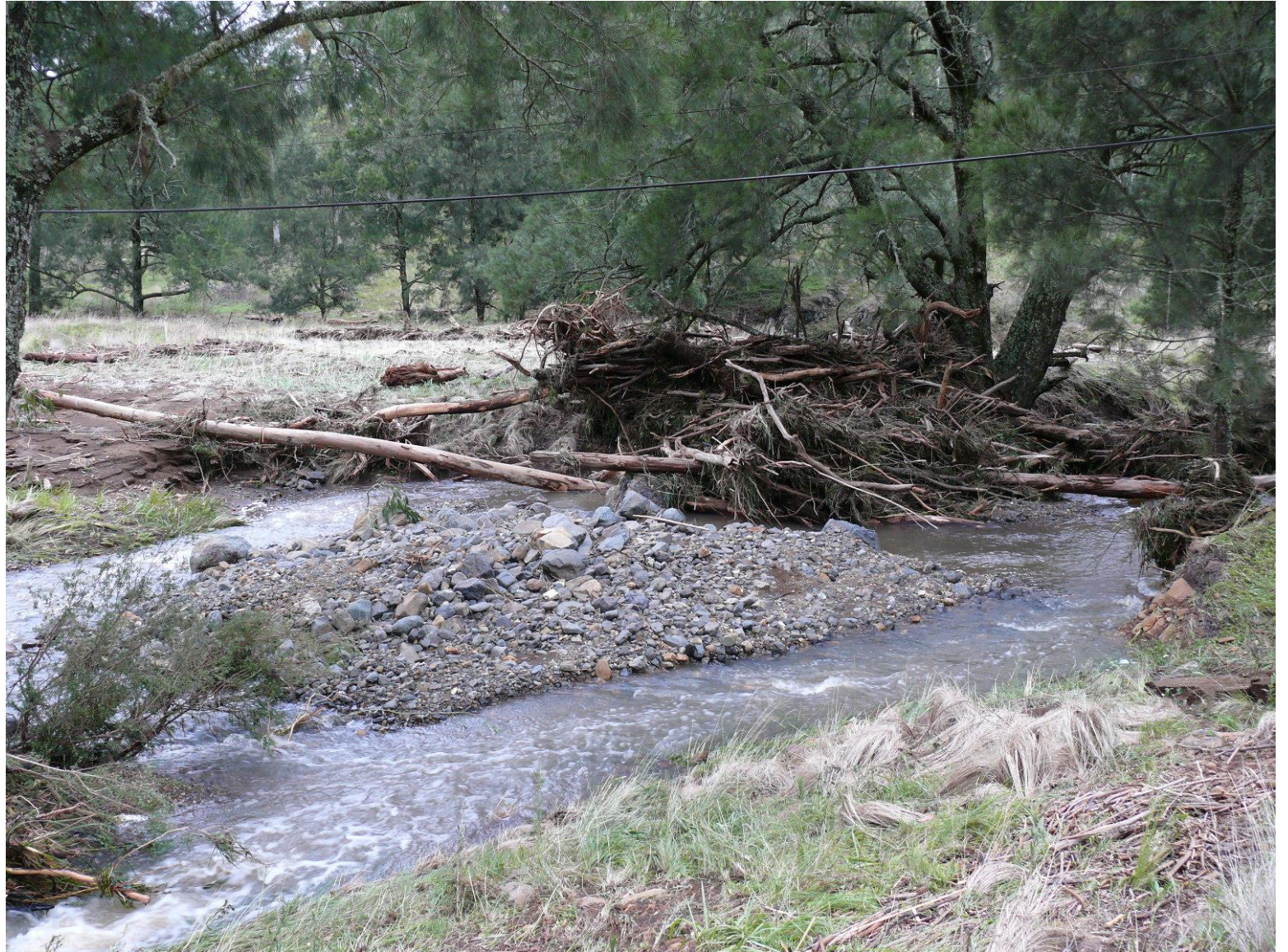
Flood debris on Shearers Road Stockyard Creek culvert after January 2, 2010 flood Stockyard Creek is a 3 rd order stream
