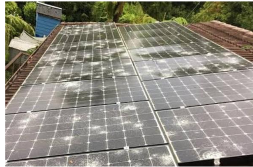
Solar panels damaged by hail
