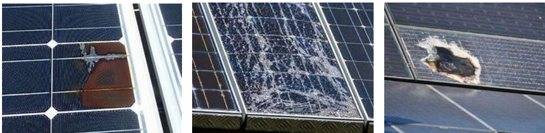
Examples of some types of PV panel deterioration
