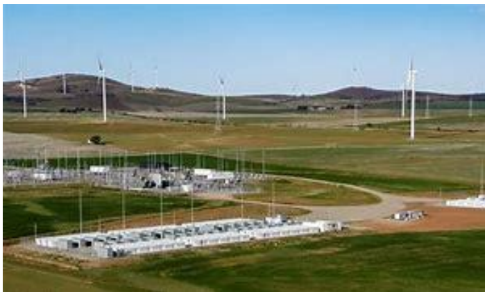
Hornsdaile Power Reserve (batteries) and Wind IEGP, South Australia
