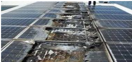
Fire shuts down whole solar array
