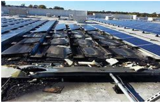
Remains of a solar panels fire
