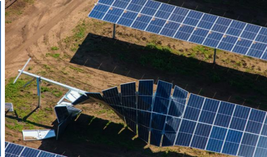
Oakey 2 wind damage
