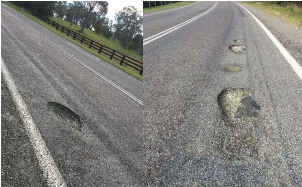
Tocal Road, pavement failure
