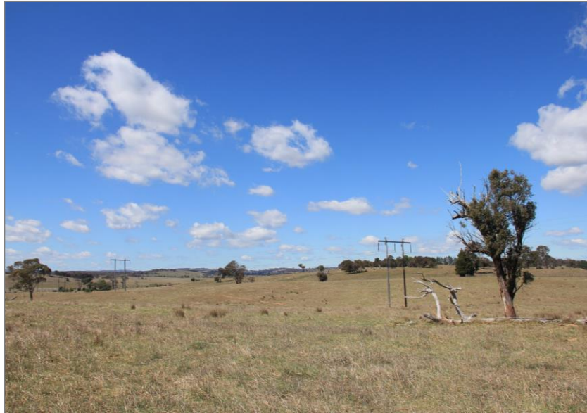
Figure 2 | Existing 132 kV transmission line infrastructure on site
