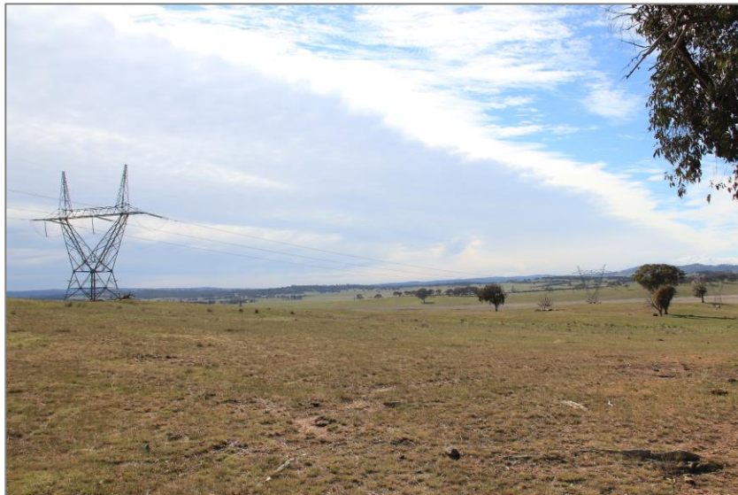
Figure 4 | Existing 330 kV transmission line infrastructure on site
