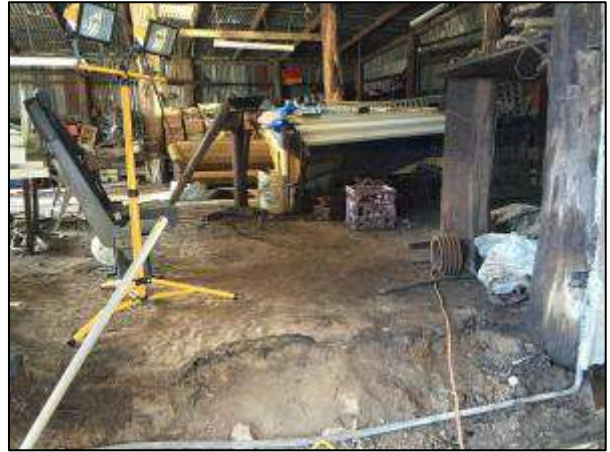
Photograph 16 – Interior of shed 3, staining observed, presumed to have been used as a workshop
