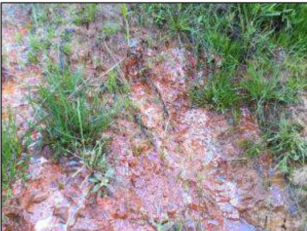
Photograph 27 – Iridescent sheen observed on water leaching from base of dam
