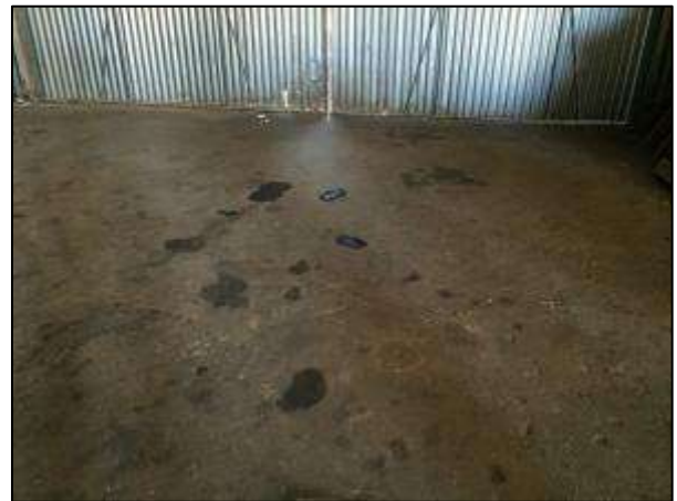
Photograph 11 – Staining present within shed 1
