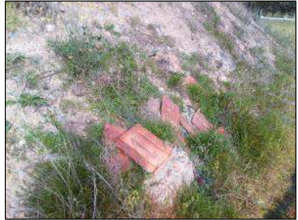
Photograph 22 – Dam wall with roof tiles and other building debris present on surface
