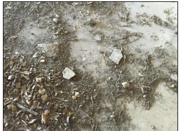
Photograph 6 – Presumed asbestos cement debris located within localised area of the former fruit shop
