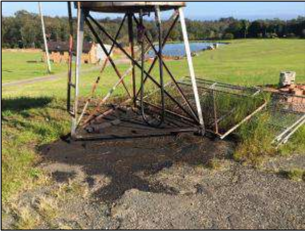
Photograph 7 – View of AST, soil staining and the cleared orchard area, facing west
