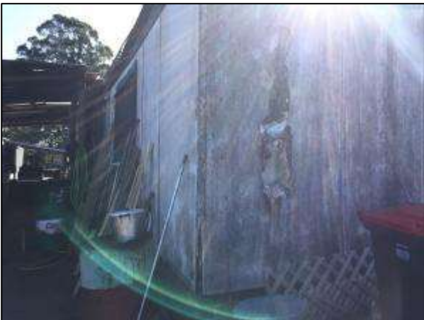
Photograph 15 – Asbestos cement sheeting in fair condition on the southern exterior of Shed 3
