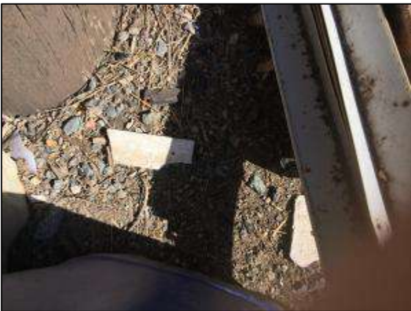
Photograph 14 – Asbestos cement debris observed on soil surface within shed 2
