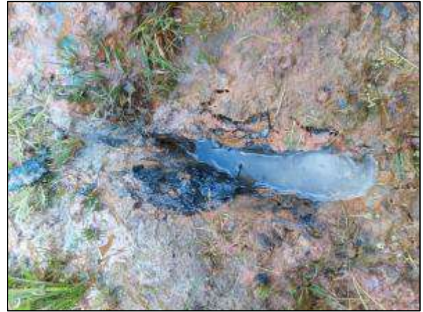
Photograph 28 – Dark black silty soil observed along the base of the dam wall
