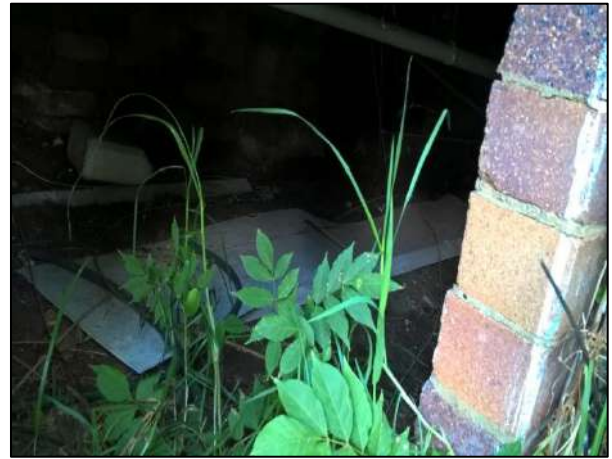
Photograph 4 – House subfloor space with presumed asbestos sheeting and debris
