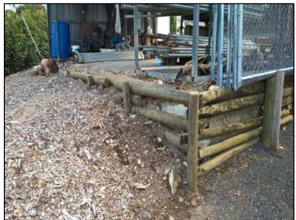
Photograph 12 – Car port in the north-western apex showing potential fill and raising.
