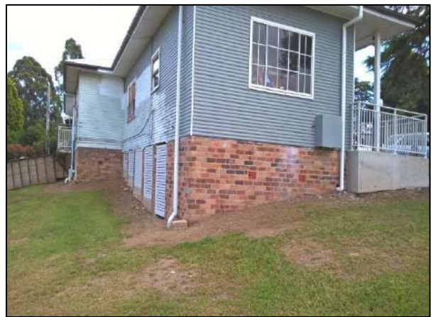
Photograph 11 – Exterior of house with disturbed soil profile with debris on surface (facing west).
