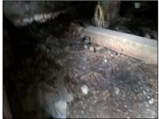
Photograph 9 – Presumed asbestos cement debris on soil surface within sub-floor space
