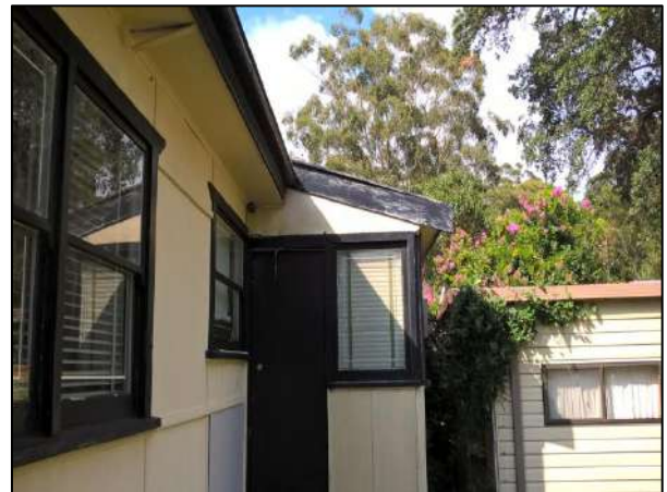
Photograph 6 – Rear of house showing presumed asbestos wall cladding (facing south)
