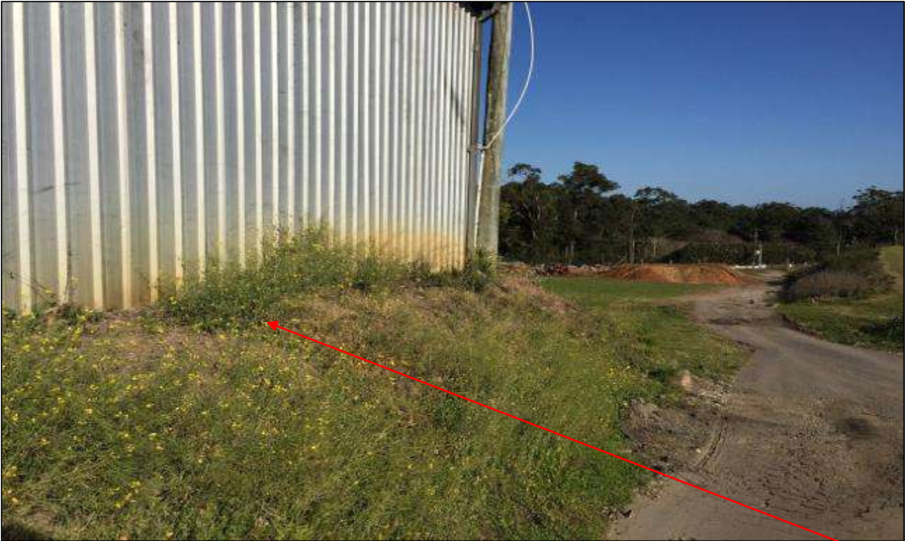
Photograph 1 – Facing west towards Derriwong Rd on the northern boundary of the site. Fill materials beneath the storage shed
