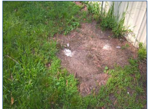
Photograph 4 – Slab present adjacent to the southern fence line in the eastern portion
