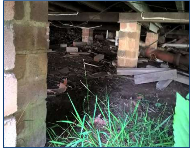
Photograph 2 – Sub-floor space of eastern house, presumed asbestos cement debris
