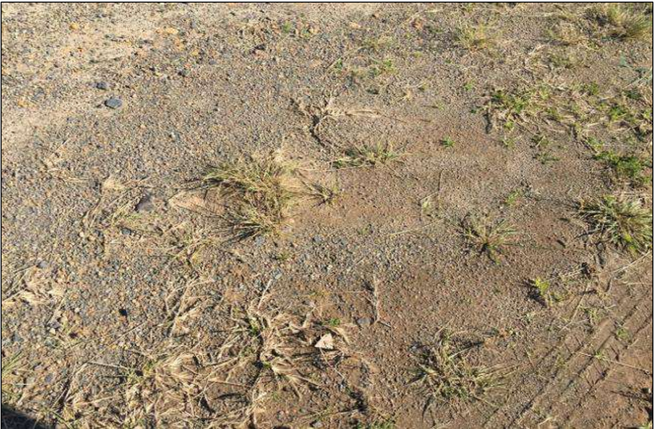
Photograph 10 – Fill materials present on the eastern boundary of the site with asbestos observed on the soil surface
