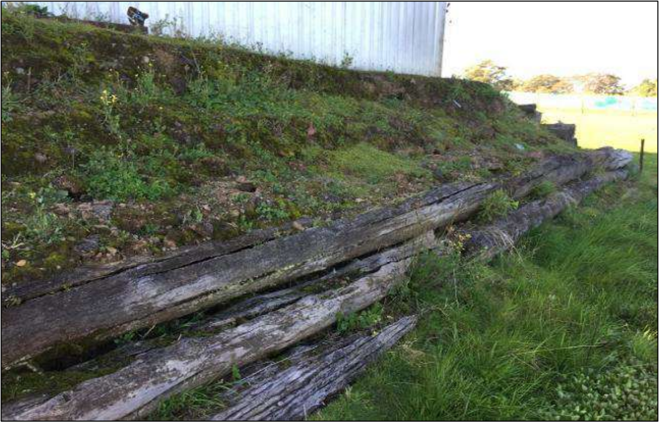
Photograph 3 – View of fill materials on the southern side of the storage shed
