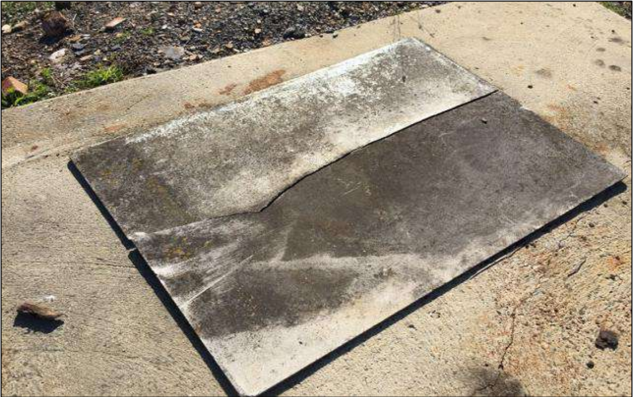
Photograph 7 – Slab located on eastern boundary of site with asbestos sheeting on surface. Small amounts of staining observed on the concrete
