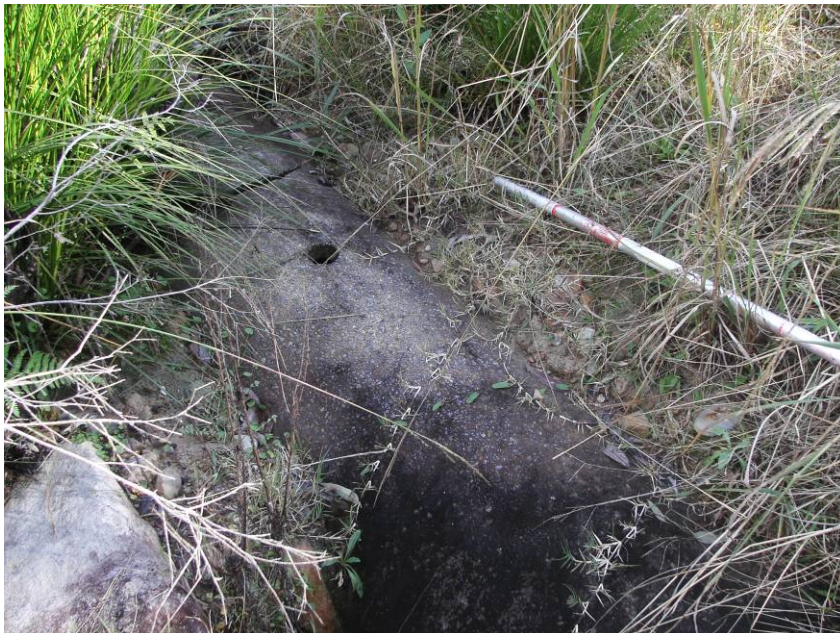
Plate 14: SU3 showing water pipe line trending in a south easterly direction - view to north west.
