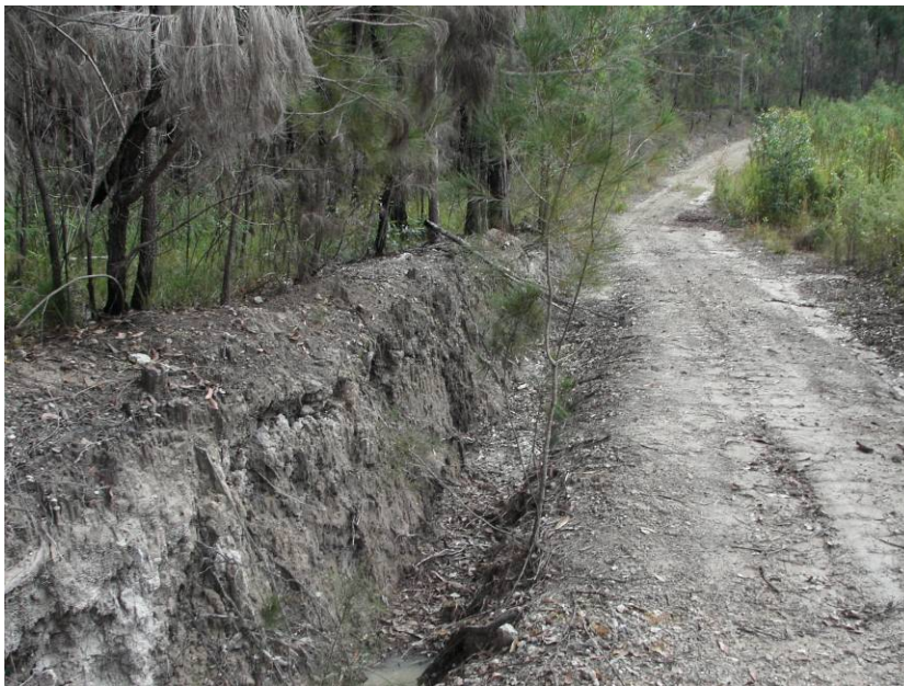
Plate 2: SU1 showing excavated drainage channels along existing dirt tracks – view to north.
