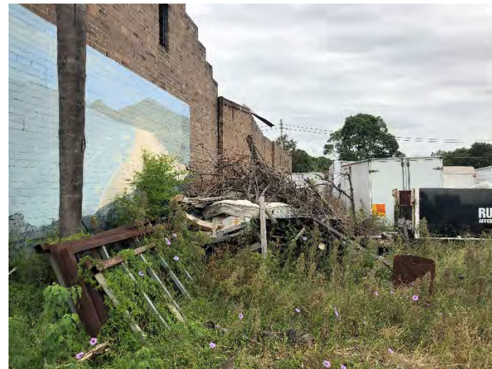
Piles of waste in leased area behind Building B and C.
