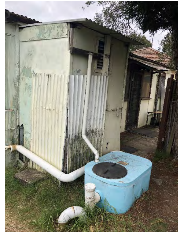
Grease trap system at the rear of the Corner Shop.
