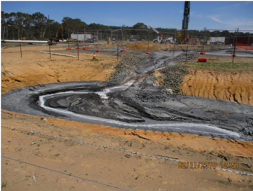
Photo 13. Run off from drilling dewatering bores on UCML's Lot 8 draining to Borrow Pit dam.
