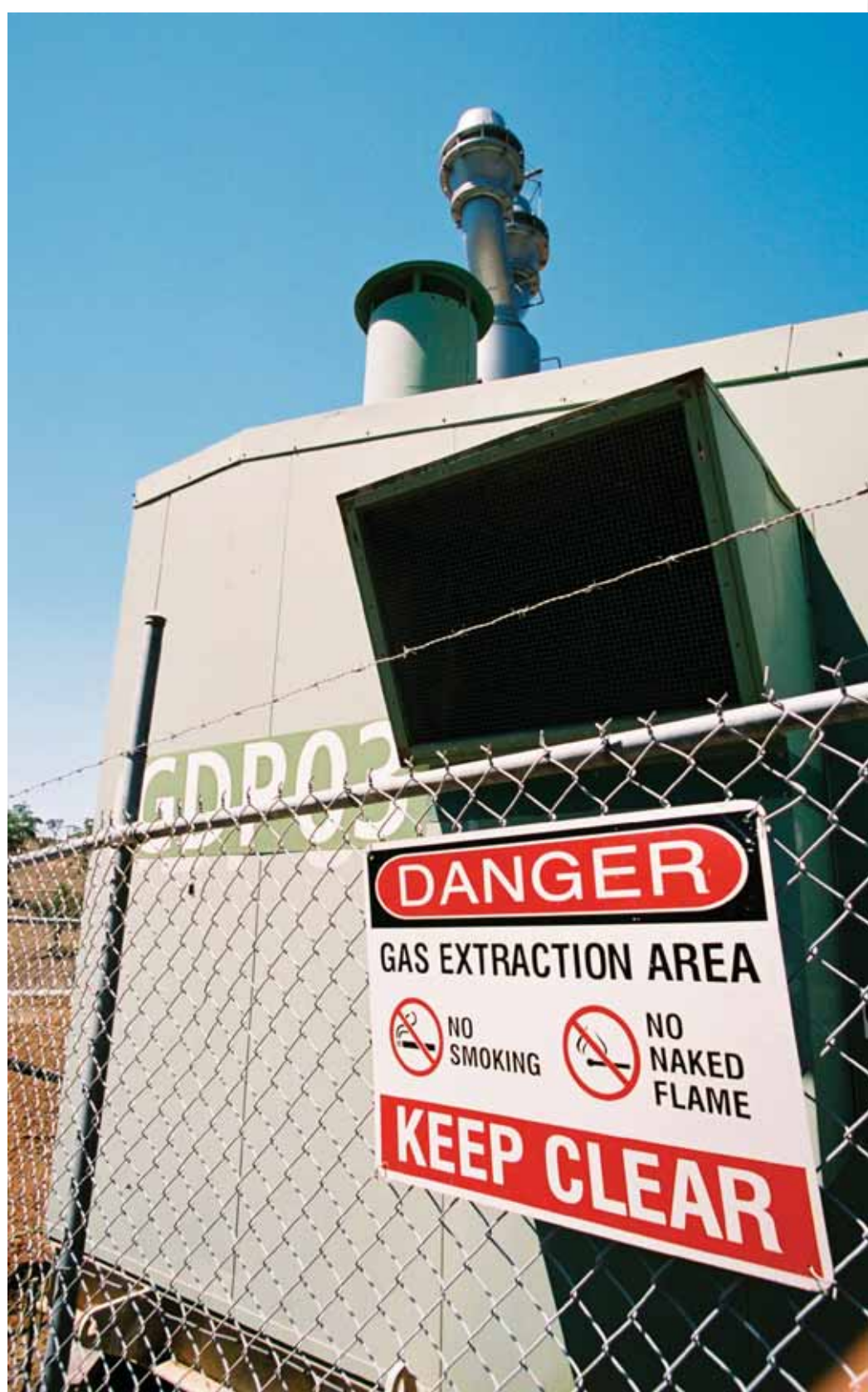
Above: Infrastructure for the methane flaring trial.
