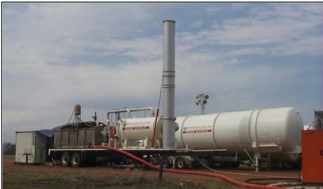
Figure 27: Mineshield inertisation unit
