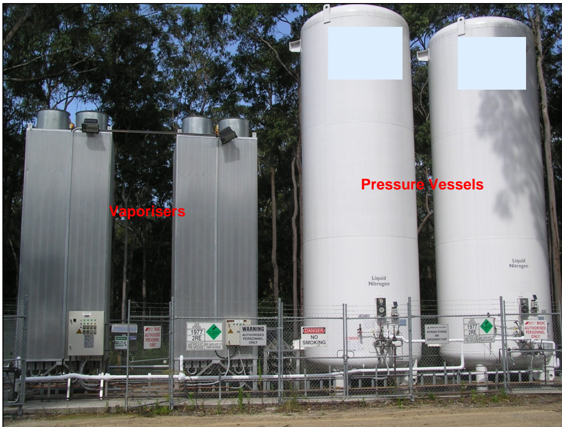
Figure 28: Ambient Air Vapouriser
