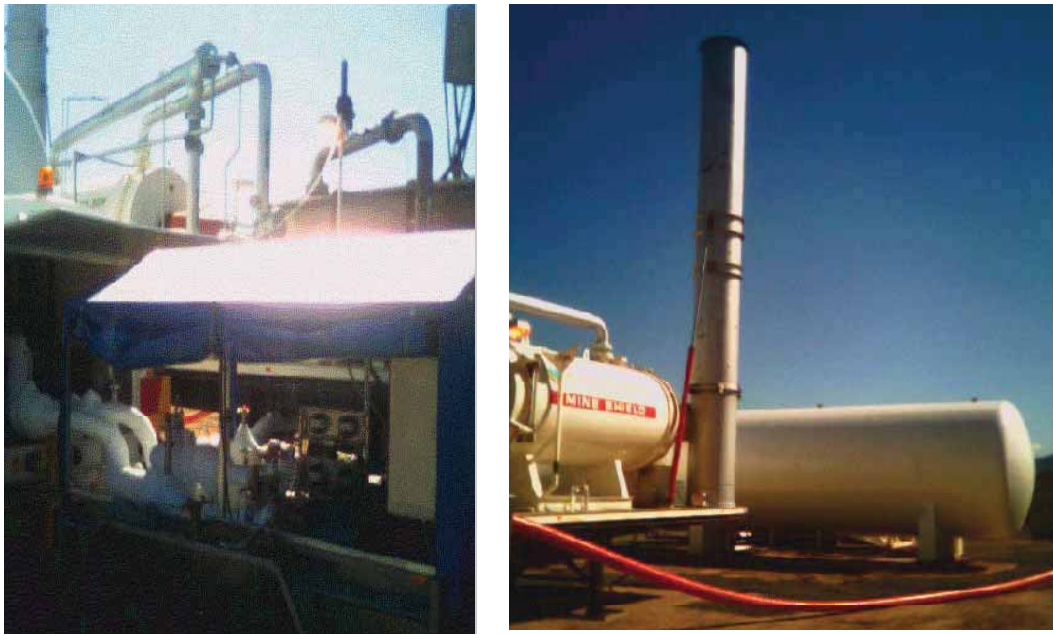
Figure 2.4 Mineshield on mine site, pump and vaporisation unit
