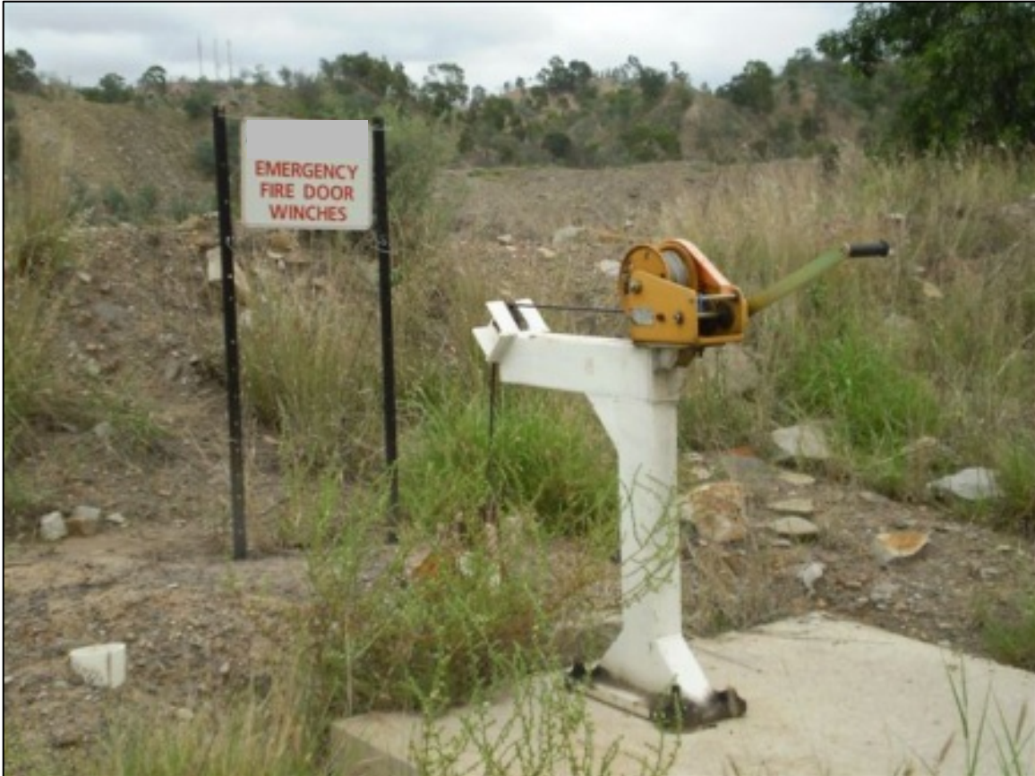
Figure 41: Surface located winch to activate door
