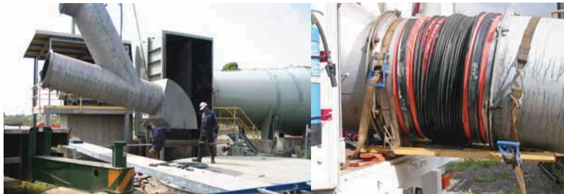
Figure 4.4 Positioned shaft cap, injection elbow and flexible elbow to GAG and aligning GAG flexible connection.
