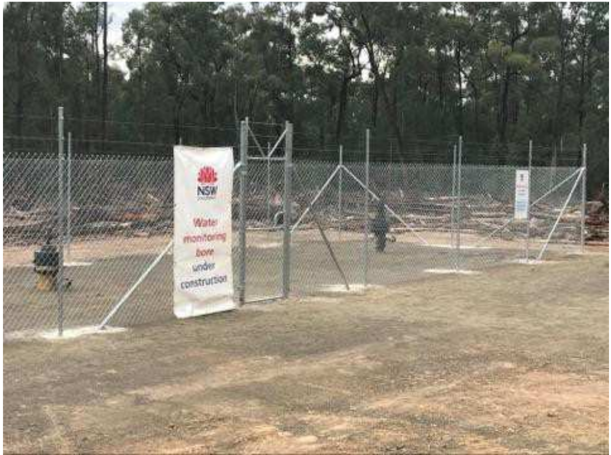
Figure 3-4: Typical site set up for water monitoring bore constructed to NSW Code of Practice for CSG Well Integrity
