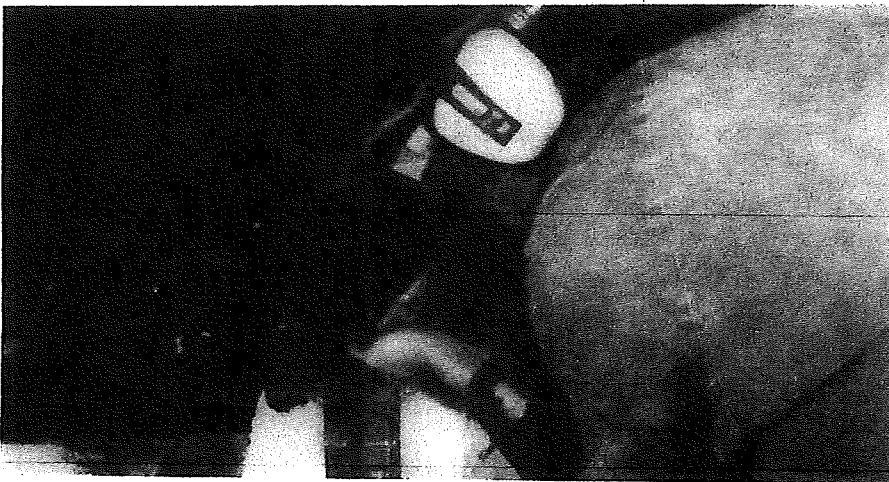
Photo 9. My assistant, Robert Bucholtz chipping a deep vee preparation prior to electric arc welding using a high nickel electrode.
