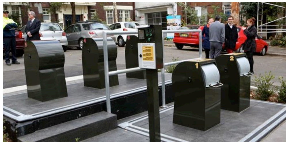
Figure 95: An underground waste storage system installed in Darlinghurst, Sydney Source: www.smartbin.com
