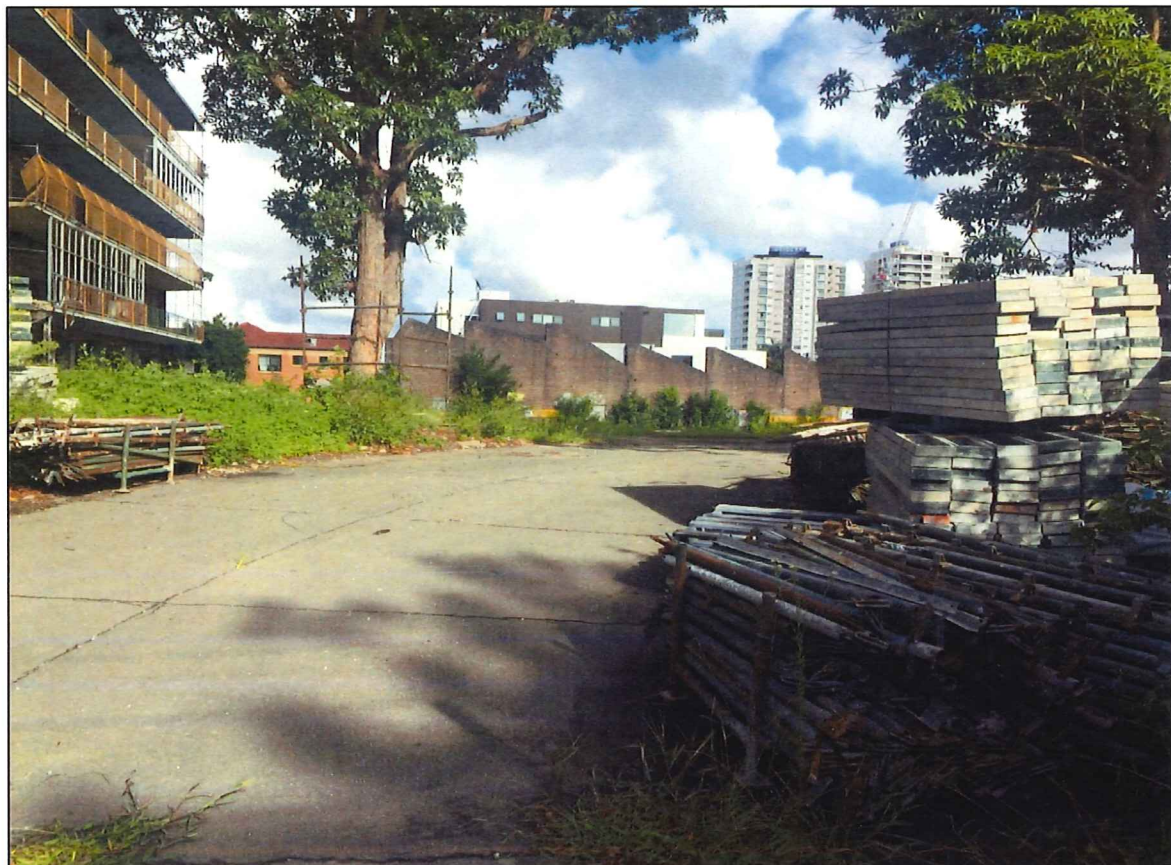
Figure 4: Existing partially excavated subject site with retained Building A to the left.
