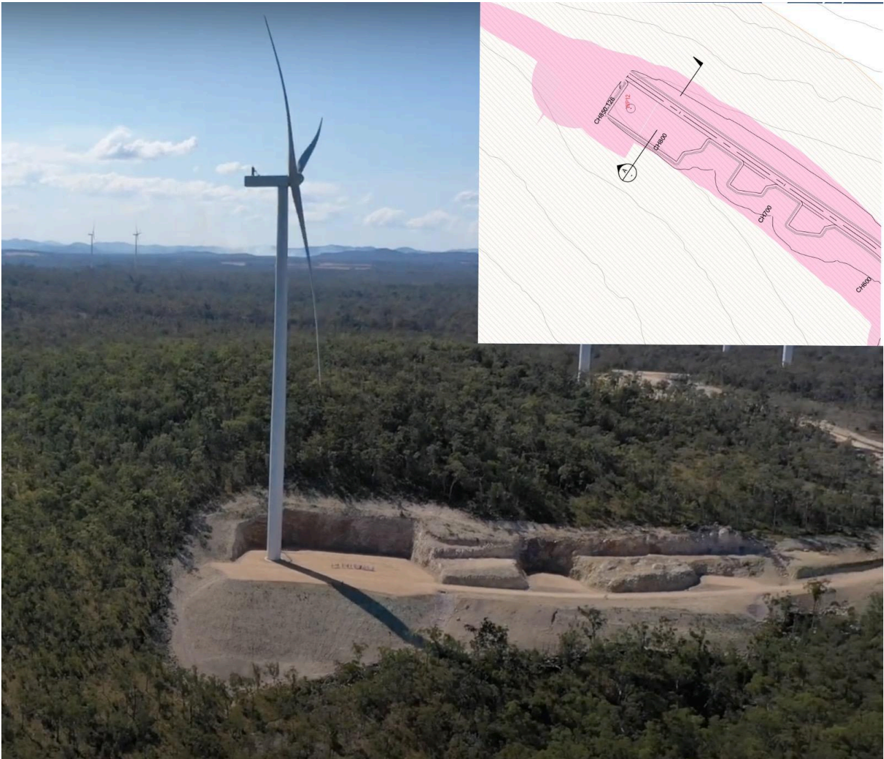
Kaban Wind Farm hard stand on narrow ridgeline with steep escarpment similar to Turbine 42. Inset, WTG 42 Layout Plan, Appendix L Constructibility Advice, Appendix B.
