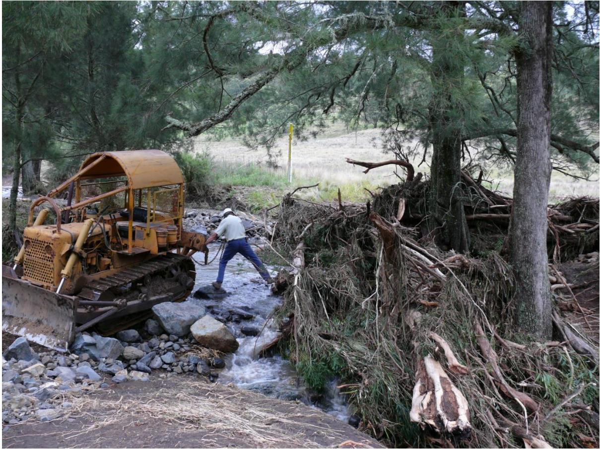
Figure 3: Flood debris deposited in Stockyard Creek/Shearers Road culvert following a 40-minute rainfall event February 2, 2010.
