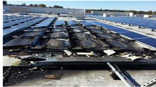
Fire damage to a PV solar IEGP
