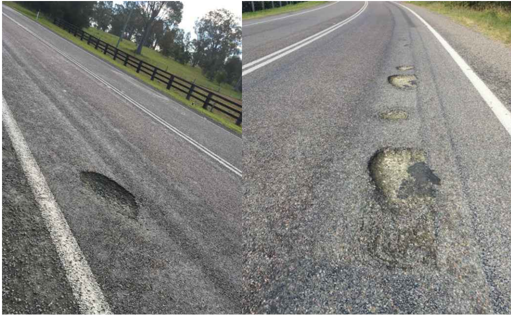
Tocal Road, pavement failure
