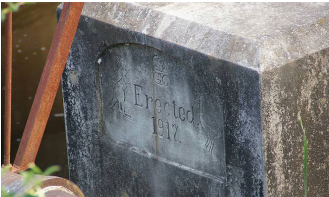
GCC imprint in the support pier Phil Hurren Jan 2016
