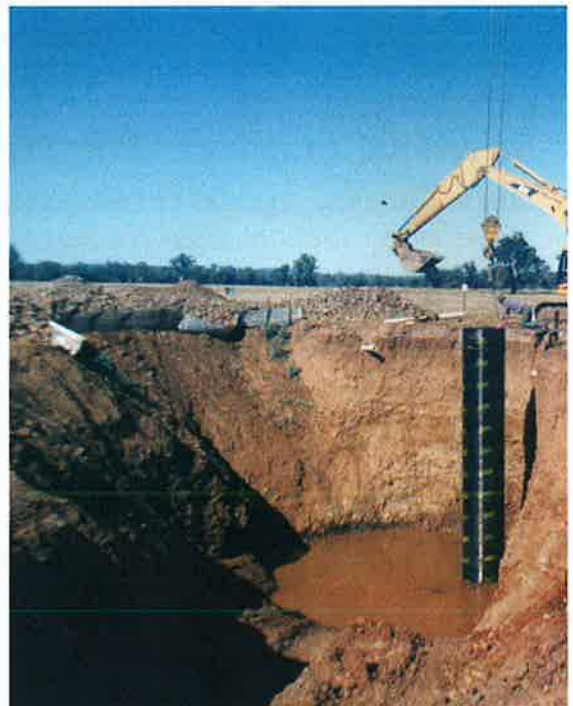
Digging out the polluted well. Note the screened rock ready to push into the hole and Cliff on a board controlling the pipe
