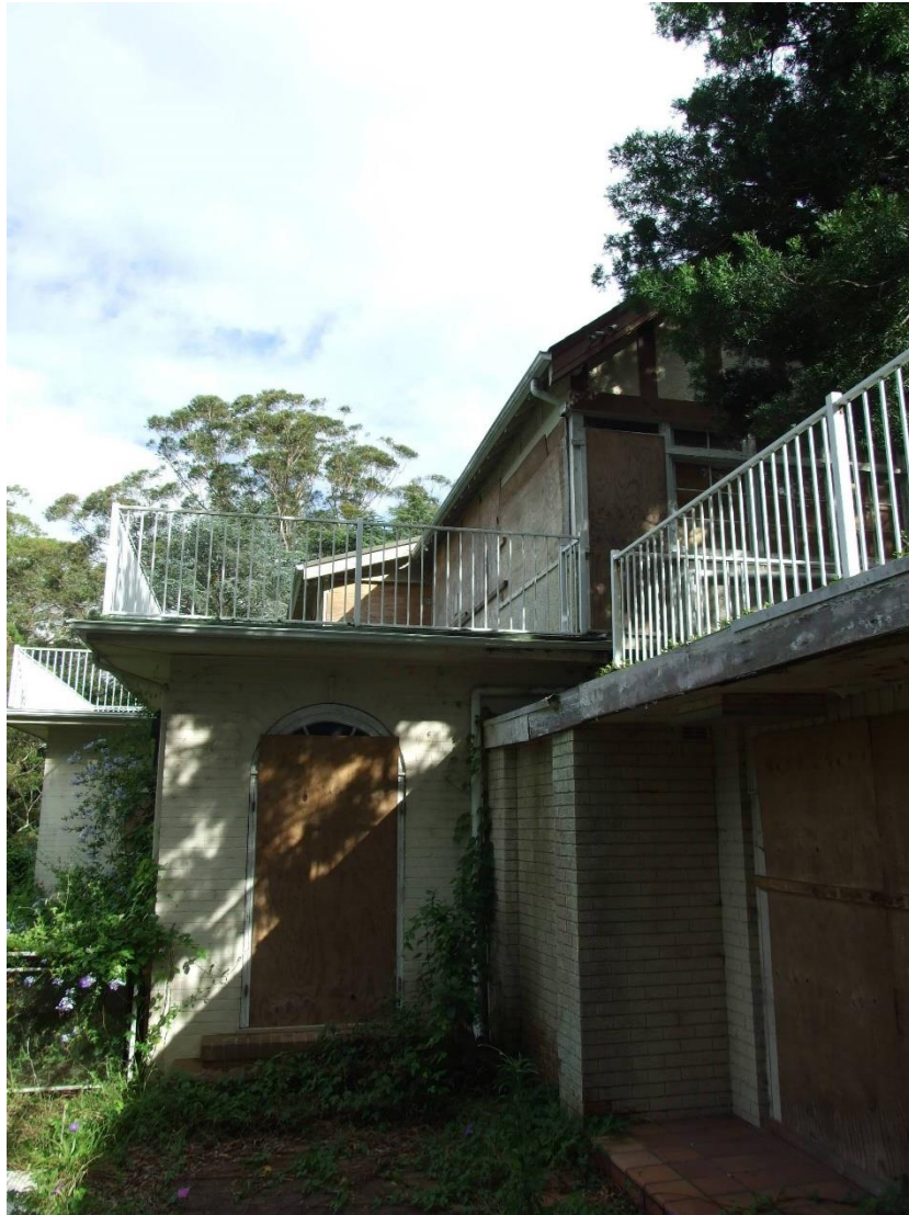
Figure7 - The modern pool house additions, flat roofed extensions and 1940s Billiard Room addition on the southern side of the house. The Pool House is proposed to be demolished to allow for new landscaping as a setting for the heritage item.
