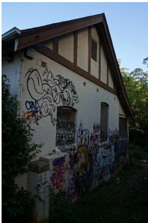
Figure 12 - Northern elevation showing graffiti and boarded up windows.
